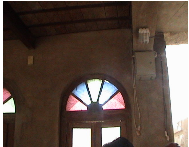
Installed Solar Controller at Dr. Mehdi's house
